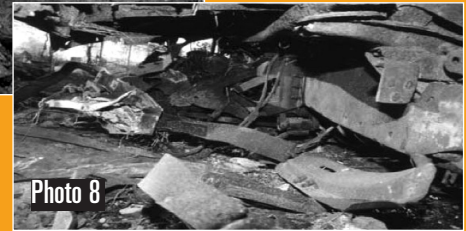
Photo 8 (below): Battery tray and support structures are damaged.
